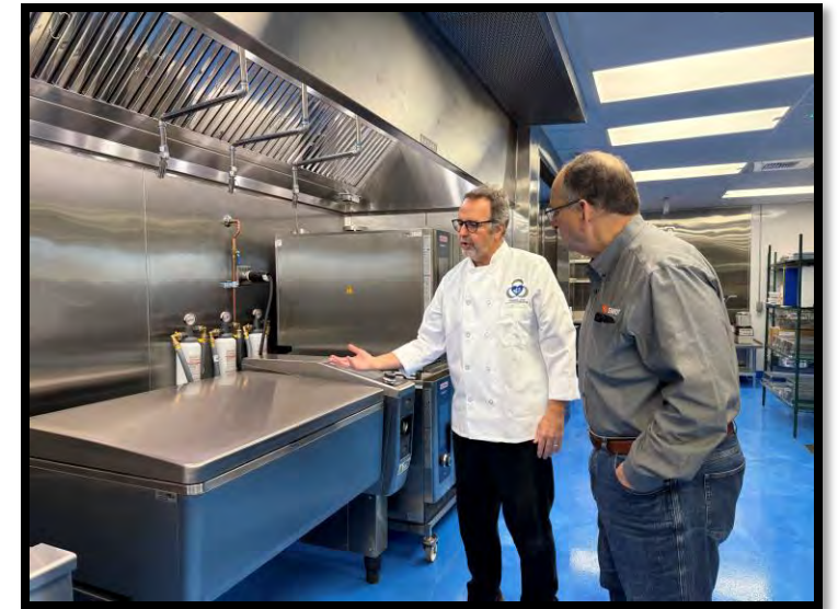
Existing Building Electrification
