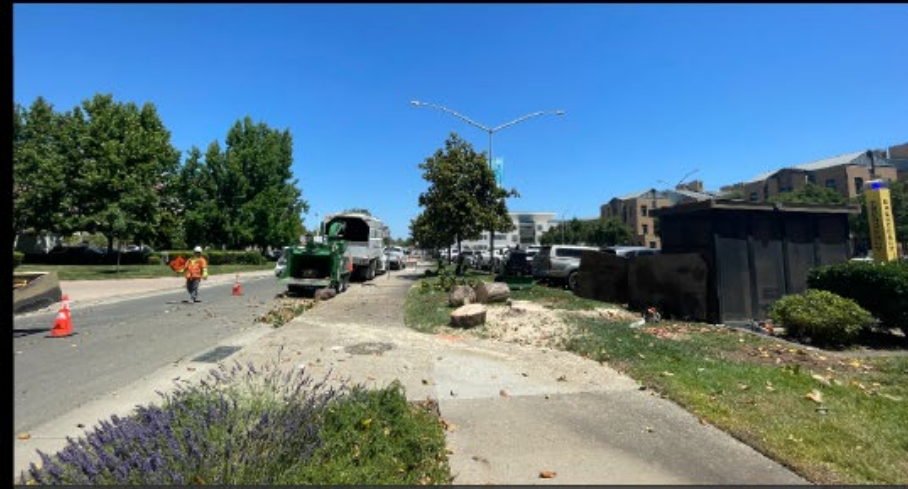
Removed Tree at the Northeast Intersection of 45th St. and 2nd Ave.
