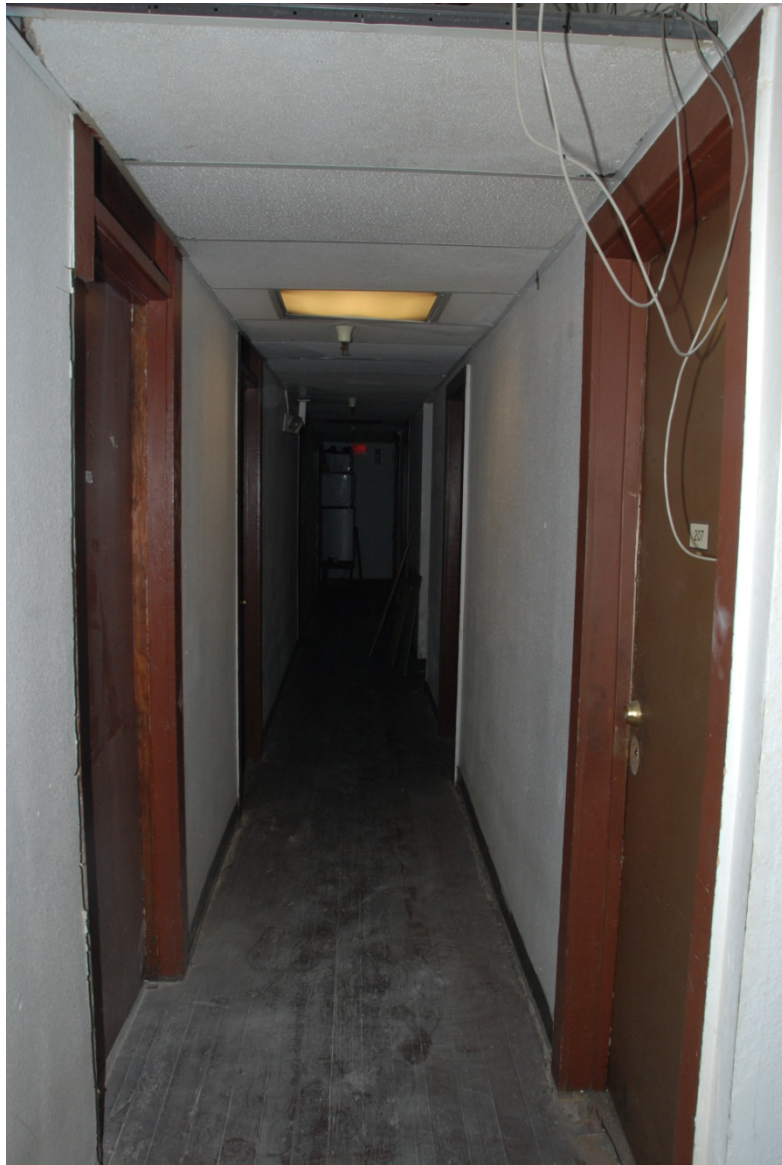
Typical hallway view. The door on left shows a partial view of the original transom molding.
