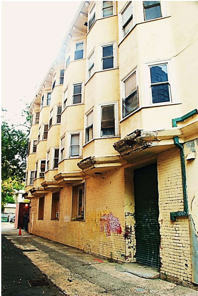
Alley elevation showing ground floor openings and banks of bay windows on upper floors. View to the northwest.
